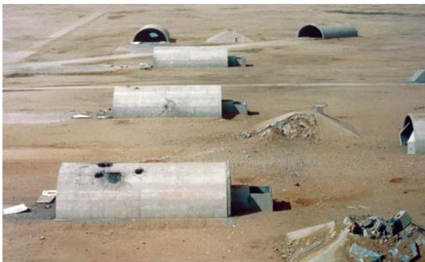
Despite Iraqi hardened aircraft shelters being constructed to the highest standards, they were no match for the 2,000lb GBU-27s used to such devastating effect by Senior Trend. Note how the doors of all six hangars have been blown out by the blast of the weapons exploding inside. (USAF)
